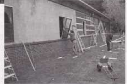
The winterizing project is designed to lower the township's cost to heat the building. Later, a stucco finish will complete the facelift.
